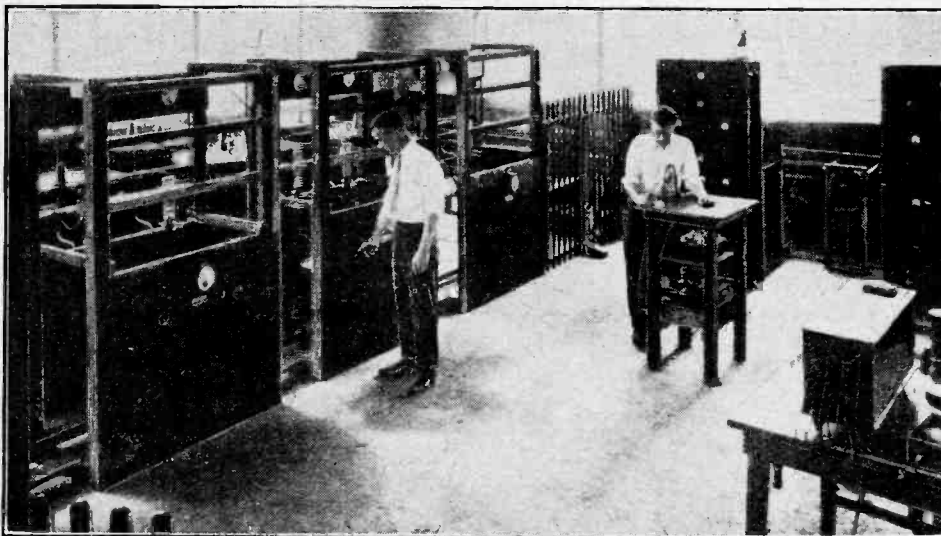
The modulating equipment. The three panels on the left each carry a group of 20 kW. water-cooled valves. The low frequency amplifier panels can be seen on the right.
